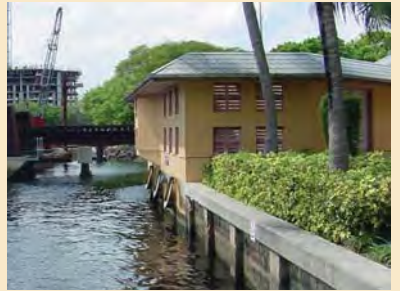
[Figure 3.36] Existing Downtown Storm Pump Station along the New River.
