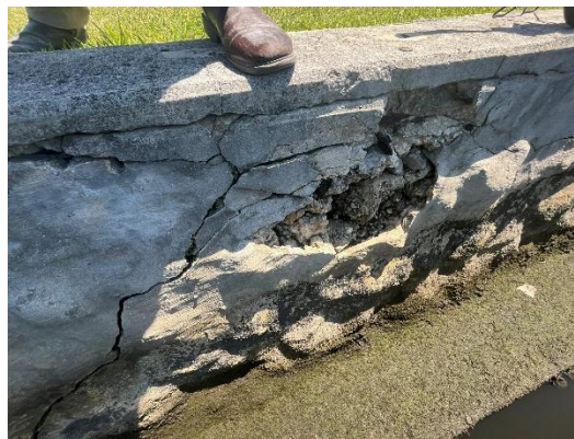
Figure 2.5.5 Missing Coral Rock in Wall (WALL 40)
