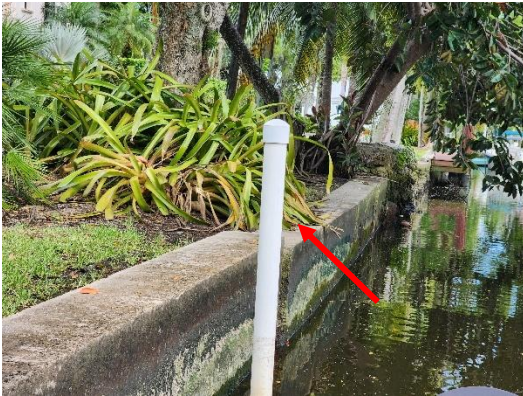
Figure 2.5.1 Lateral Movement/Rotation (WALL 27)
