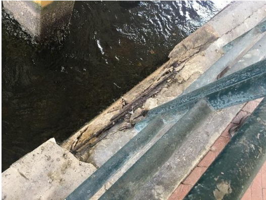
Figure 2.5.3 Typical Spall at Cap (WALL 24)
