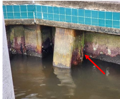
Figure 2.5.4 T-Pile and Batter Pile Spall (WALL 41)
